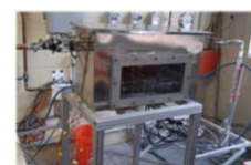
10 kW 2PIC Facility (ACT)
